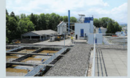
Wastewater treatment facility REAL, 6032 Emmen; Video report on www.jahresbericht.klik.ch
