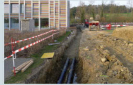
Programme participant: Wastewater heat recovery ARA Schönau - Hofmatt residential development, 6330 Cham
